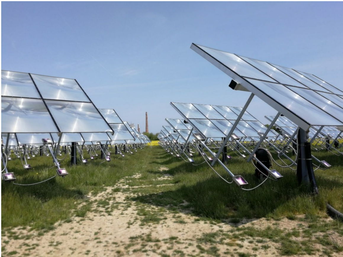
Two axis tracking concentrating solar collectors at Lendemarke solar heating plant. (DTU)
