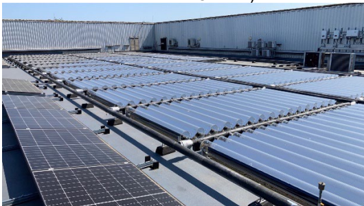
VirtuHOT collectors from Naked Energy sharing roof space with PV modules (Naked Energy. "Westgate Leisure Centre.")
