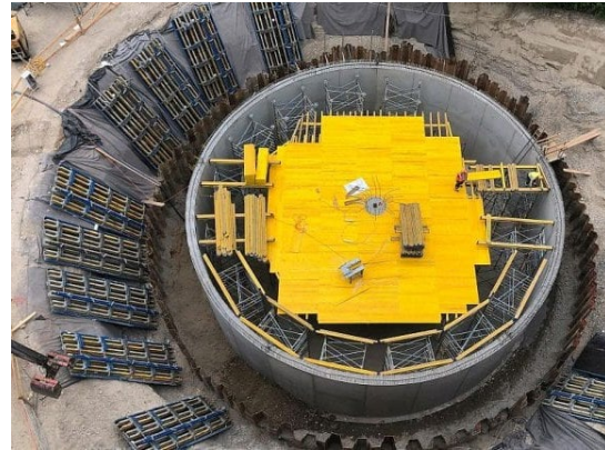
Ice store under construction with a volume of 560 m 3 for supplying heating and cooling to an urban district (Source: https://www.cleantinking.de/eisspeicher-sorgt-fuer-kaelte-und-waerme-im-quartier/ )
