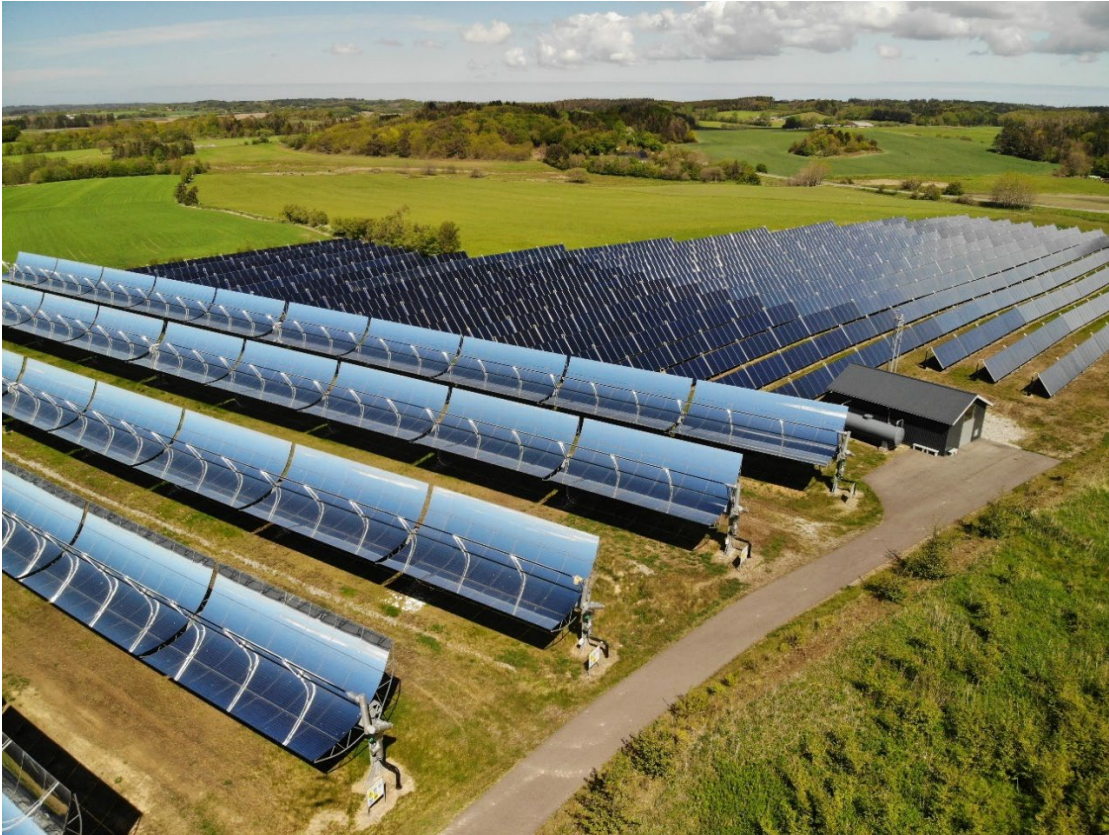
Flat plate collectors with one and two cover plates and one axis tracking concentrating solar collectors at Tårs solar heating plant. (DTU)
