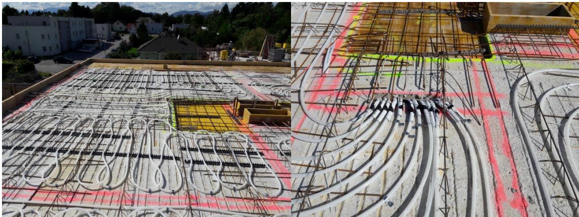
Figure: Installed TABS system before pouring concrete. The pipes for component activation are usually installed on the first reinforcement level of foundation slabs or suspended ceilings. Picture source: AEE INTEC
