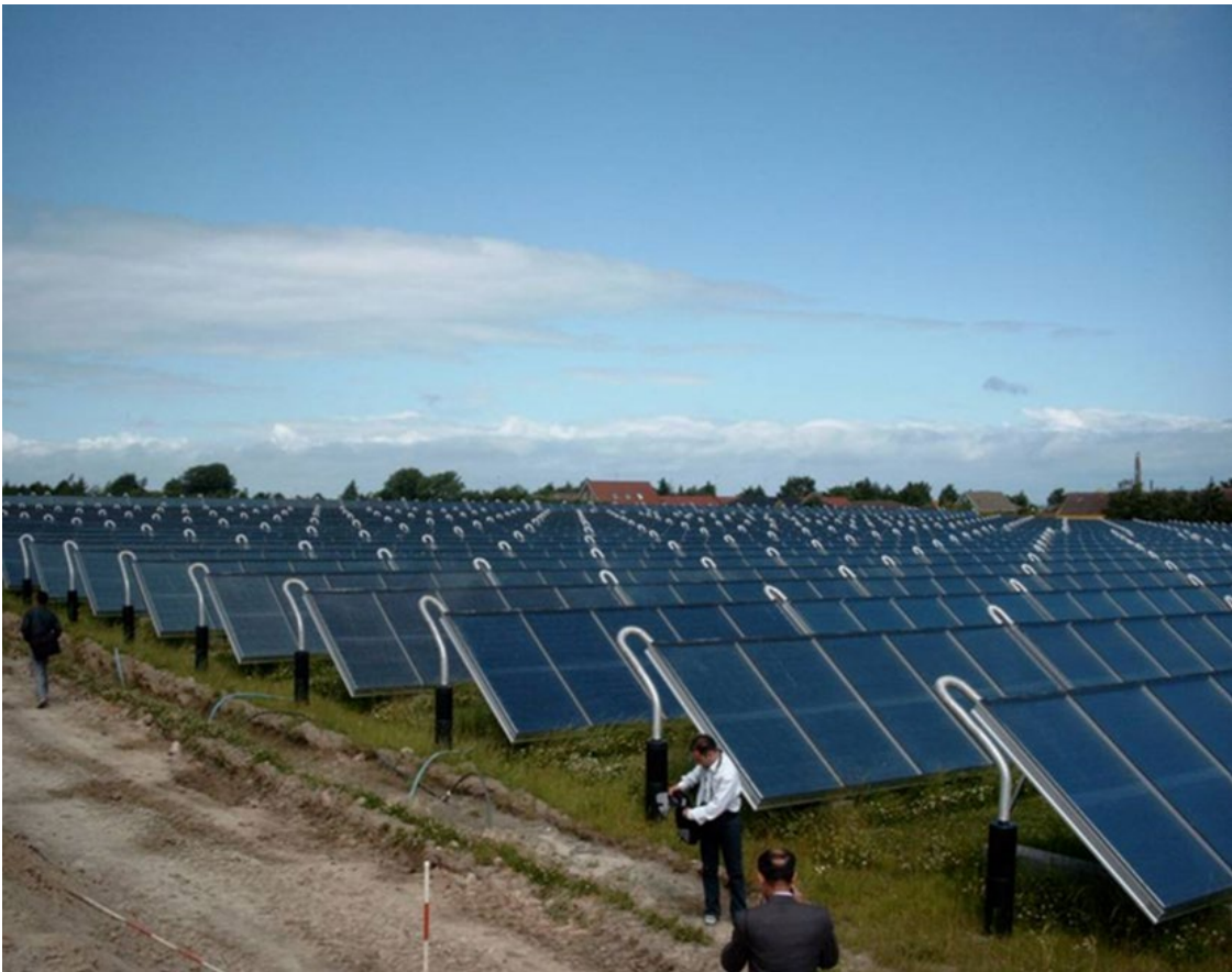
Solar collector rows at Marstal solar heating plant. (DTU)
