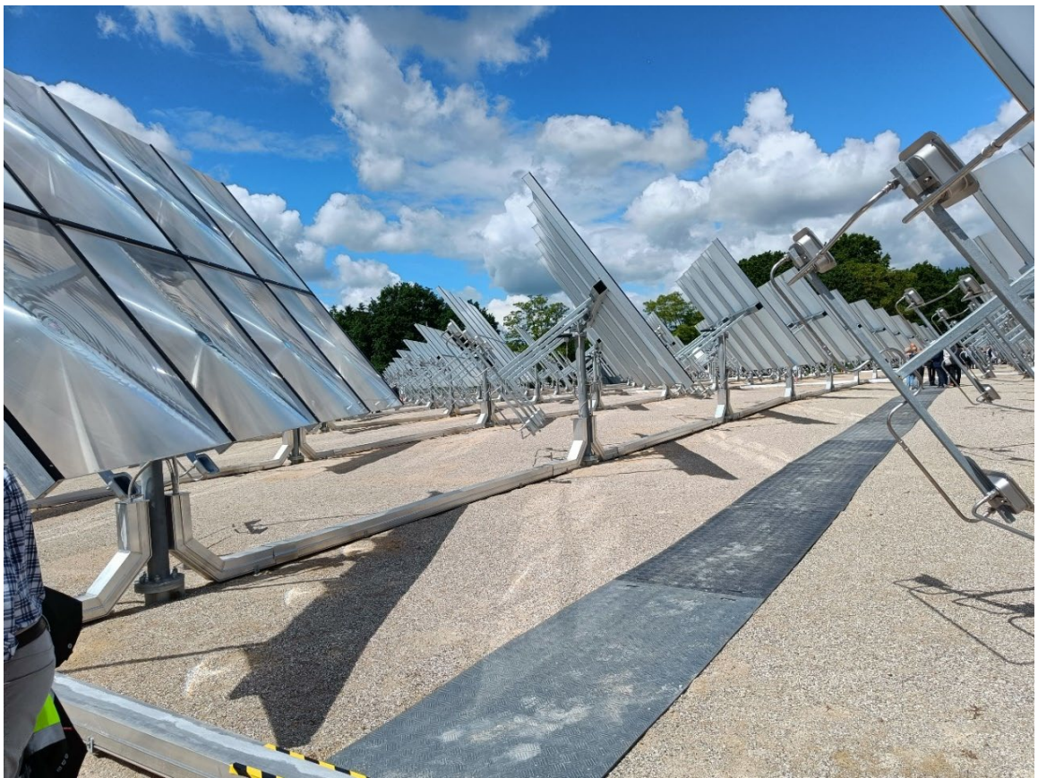
Two axis tracking concentrating solar collectors at Hørsholm solar heating plant. (DTU)
