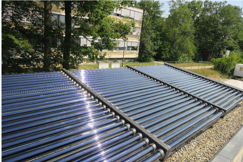
Evacuated tube air collector (airwasol) installed on the roof of the research building at the University of Stuttgart (Source: Institute for Building Energetics, Thermotechnology, and Energy Storage at the University of Stuttgart)
