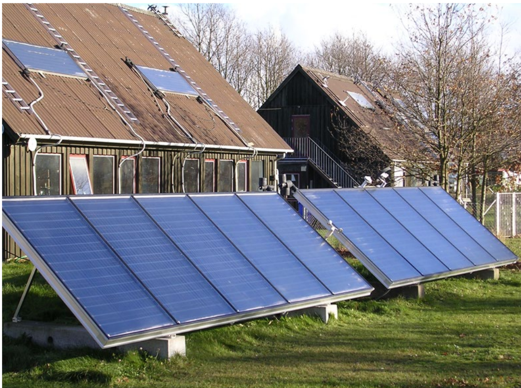
Large flat plate solar collectors under development/test at the Technical University of Denmark. (DTU)
