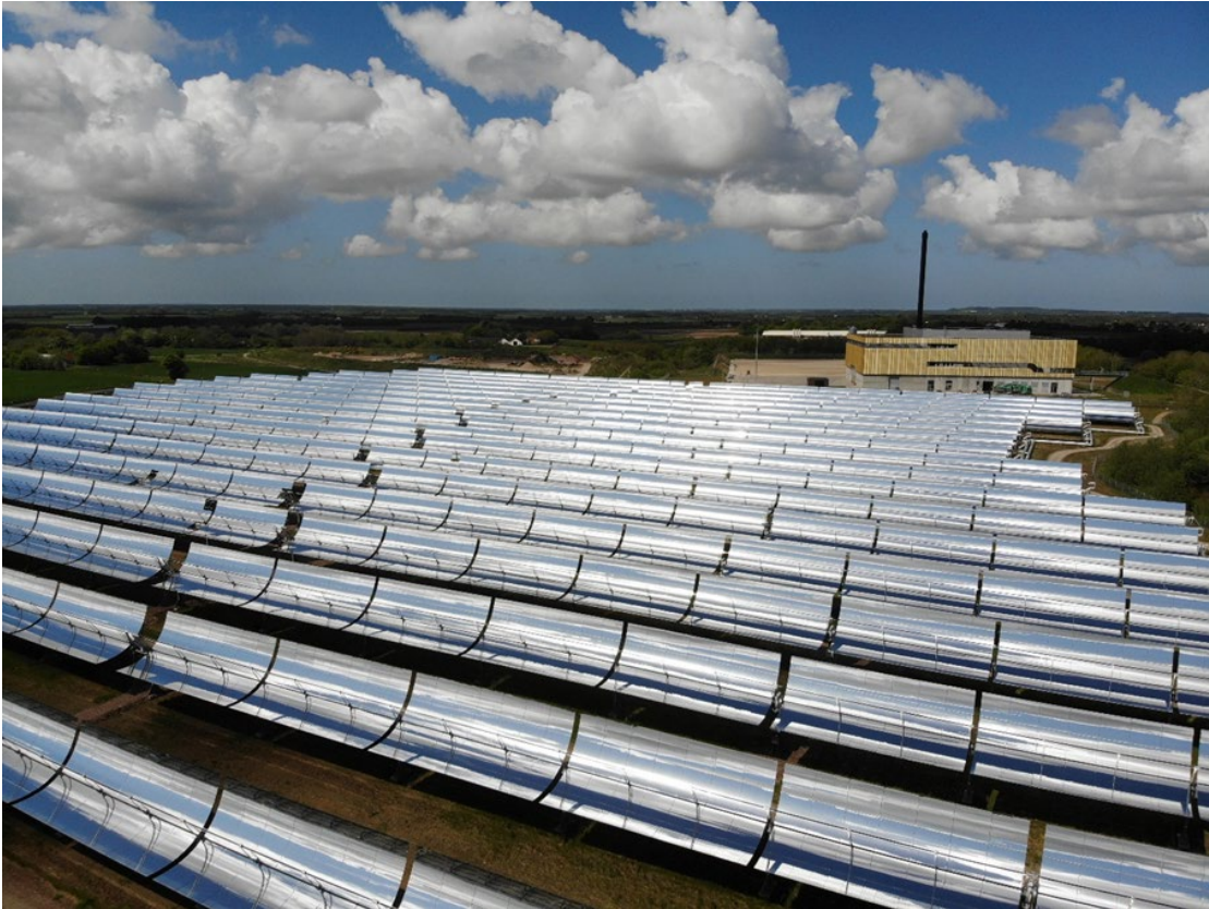
One axis tracking concentrating solar collectors at Brønderslev solar heating plant. The plant is used for both district heating and electricity production.(DTU)
